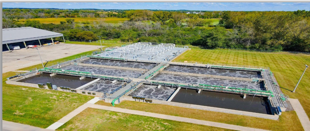
Aeration Basins and Covered Digesters
