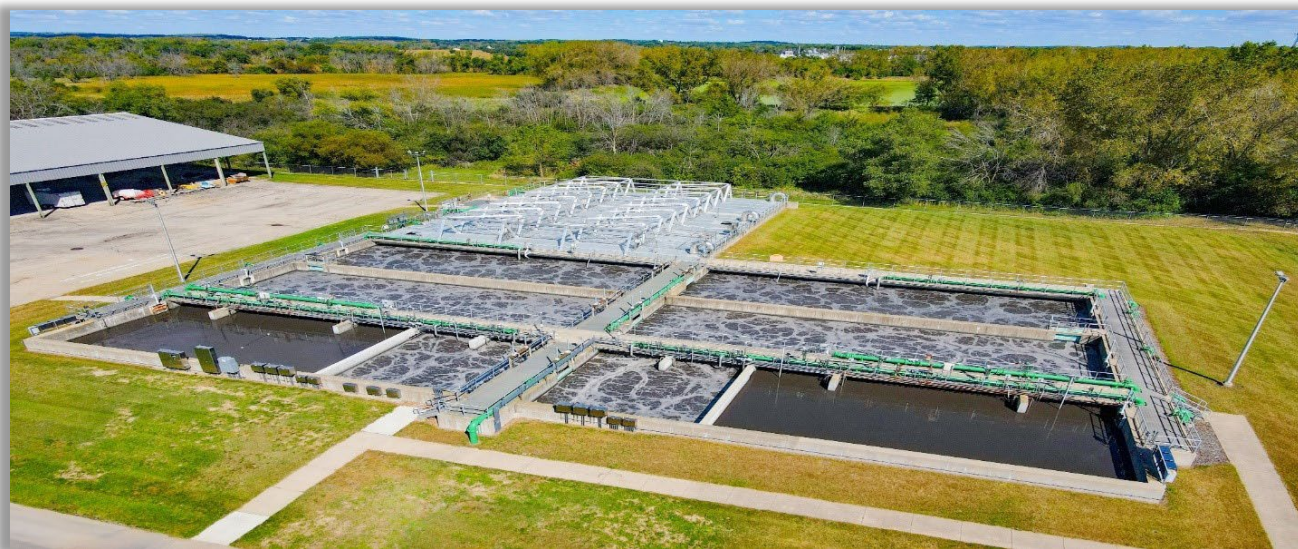
Aeration Basins and Covered Digesters
