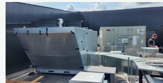
MECHANICAL, ELECTRICAL, PLUMBING, TECHNOLOGY
